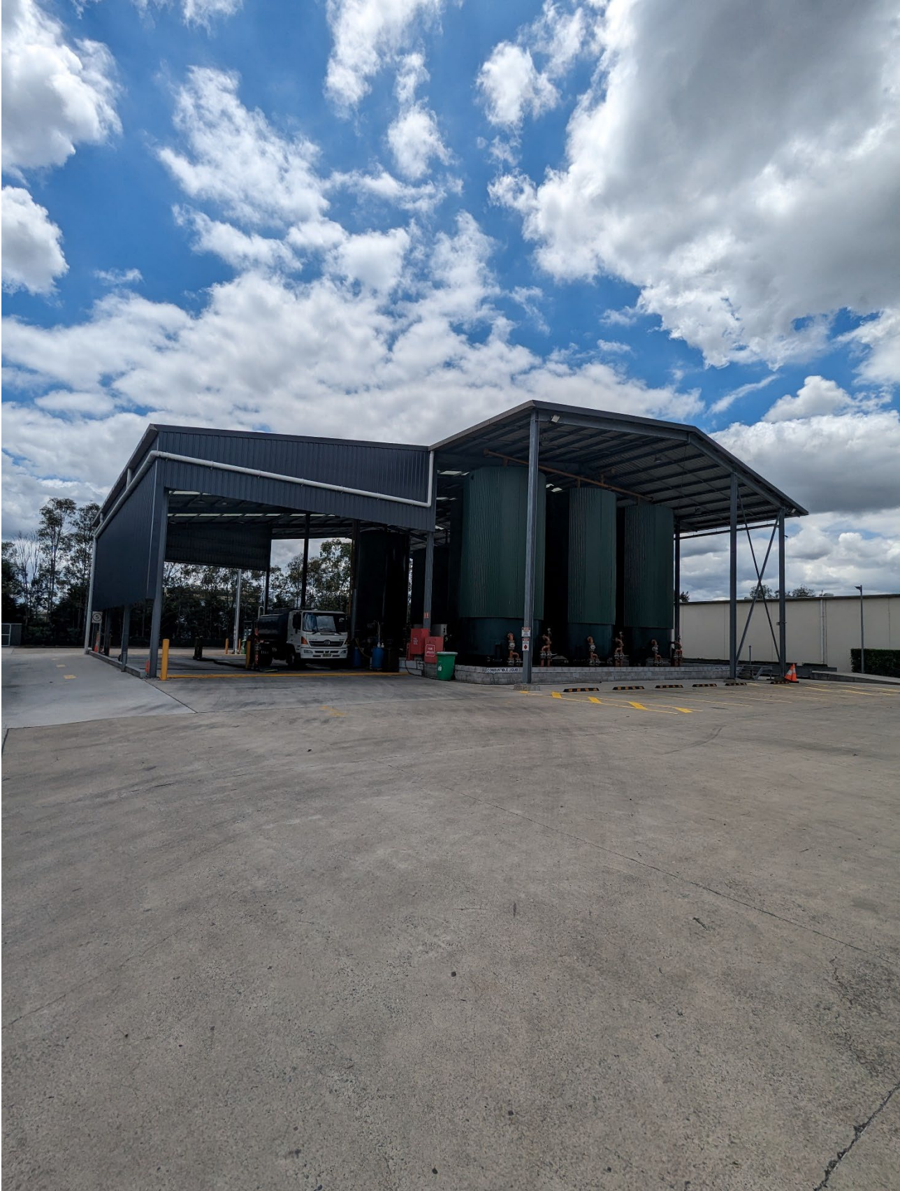
Figure D2. Photograph of the used oil banded tank farm and loading/unloading bays.
