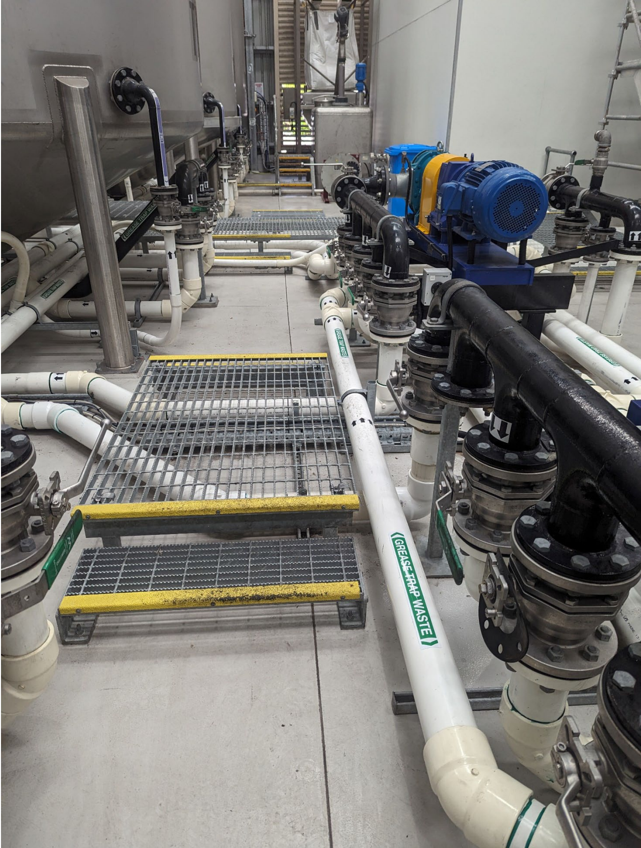
Figure D5. Photograph of floor area of the grease trap and food waste tank farm.
