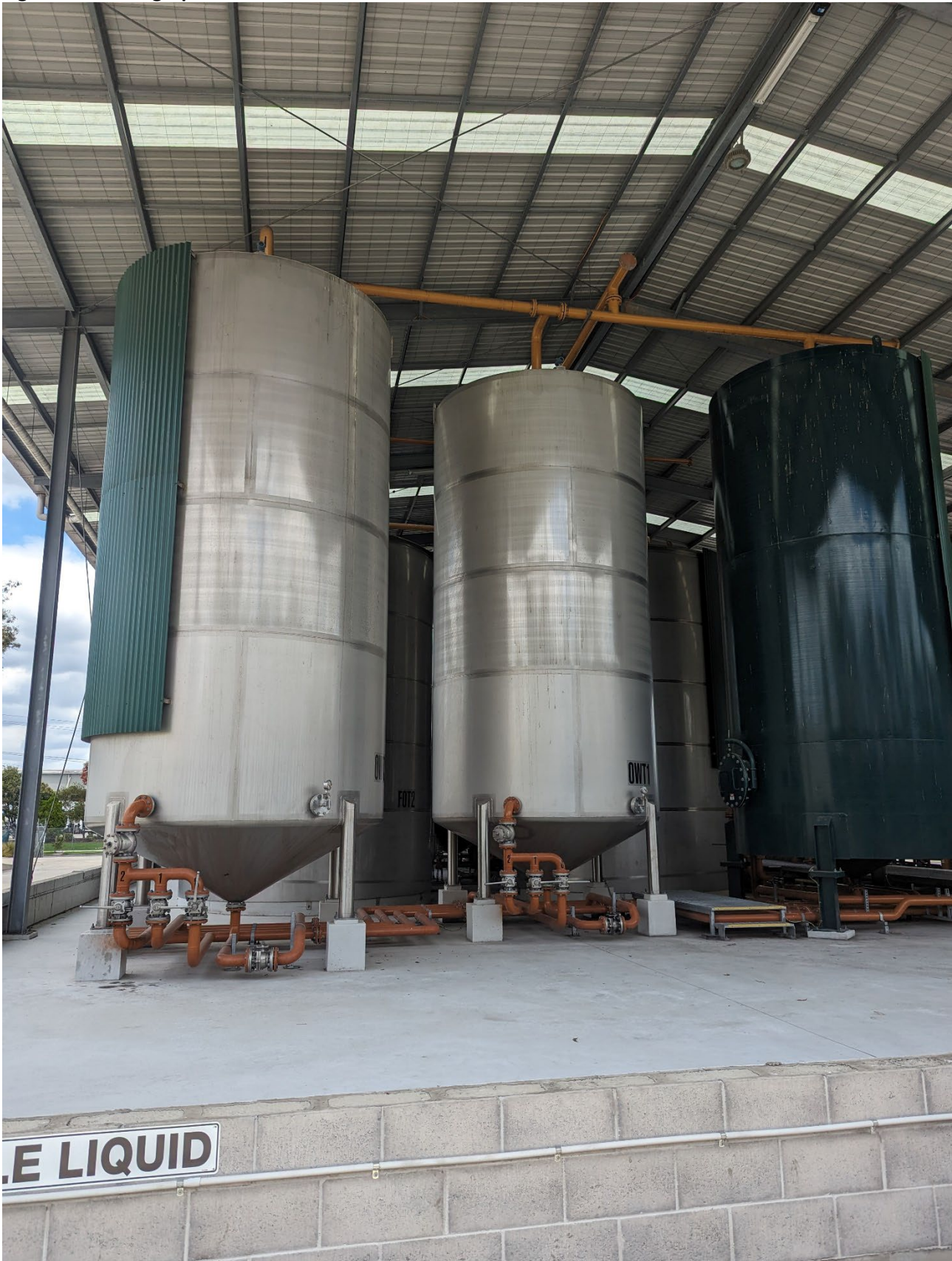
Figure D8. Photograph of the used oil banded tank farm.
