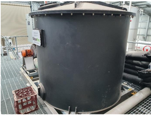
Odour Control Unit
