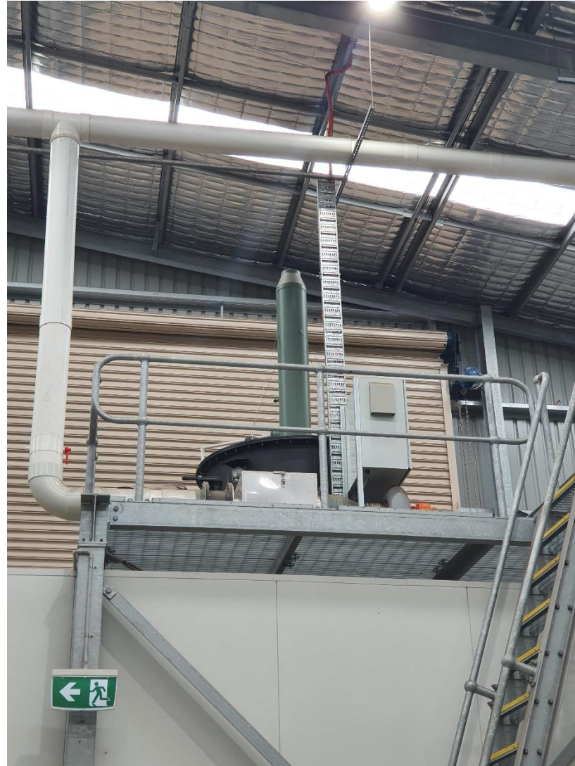
2021 Independent Environmental Audit – Glendenning Liquid Waste Facility | 78 Figure 8. Carbon filter odour control unit on top of the enclosed Dissolved Air Flotation Unit within the Organic Waste Building.
