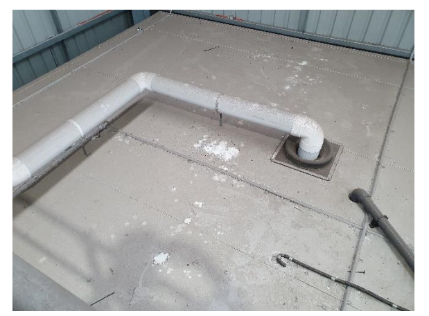
OCU connection to DAF enclosure
