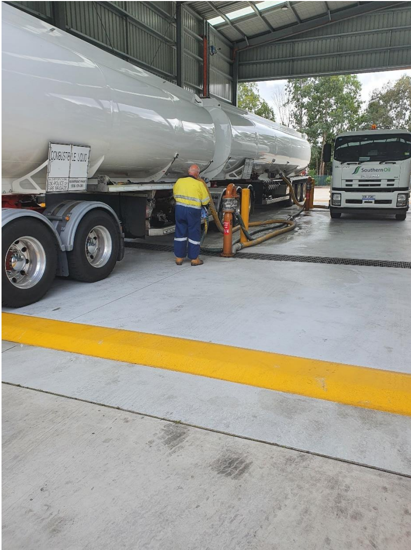
Figure 5. Loading and unloading of used oil and J120 industrial oily water is undertaken in the bunded area of the Used Oil Roof Structure.
