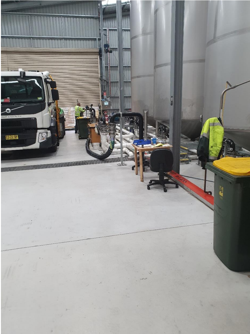
Figure 7. Loading and unloading of liquid grease trap is undertaken in the bunded area within the Organic Waste Building. Roller doors remain closed during unloading to maintain negative pressure for odour control.
