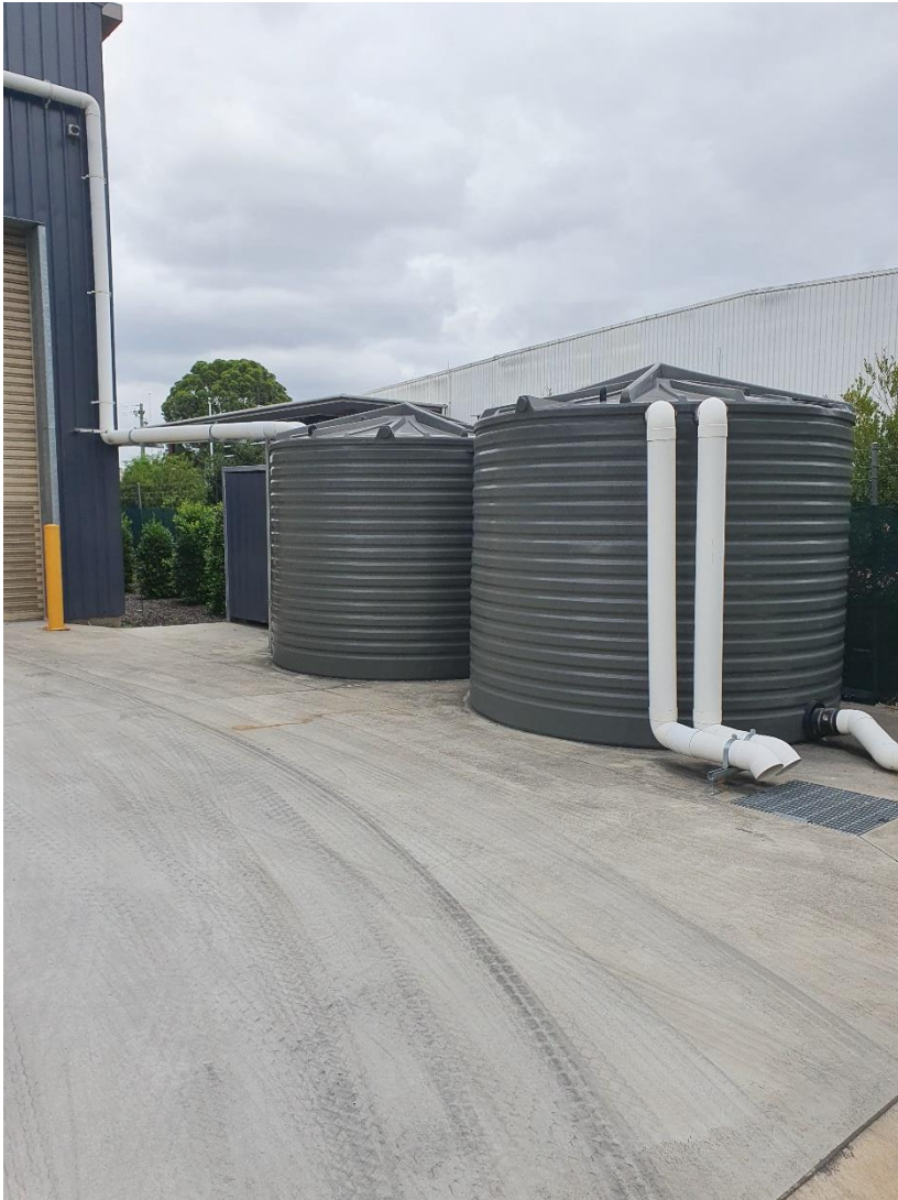
Figure 11. Rainwater capture system.
