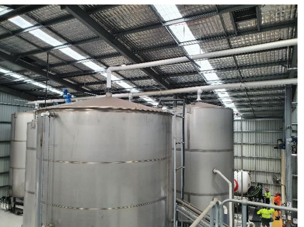
OCU connection to tanks
